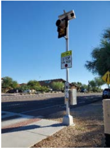
Figure 18: Existing Flashing Beacon at Ridgeview Place and Tom Darlington Drive
